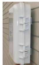
FTB/FDB in the building
