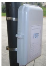
FTB/FDB on the pole
